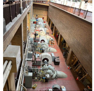
Most of these pumps date to 1928 and have been kept operating via heroic engineering and parts fabrication efforts. The WMRD is ComEd's largest customer!
